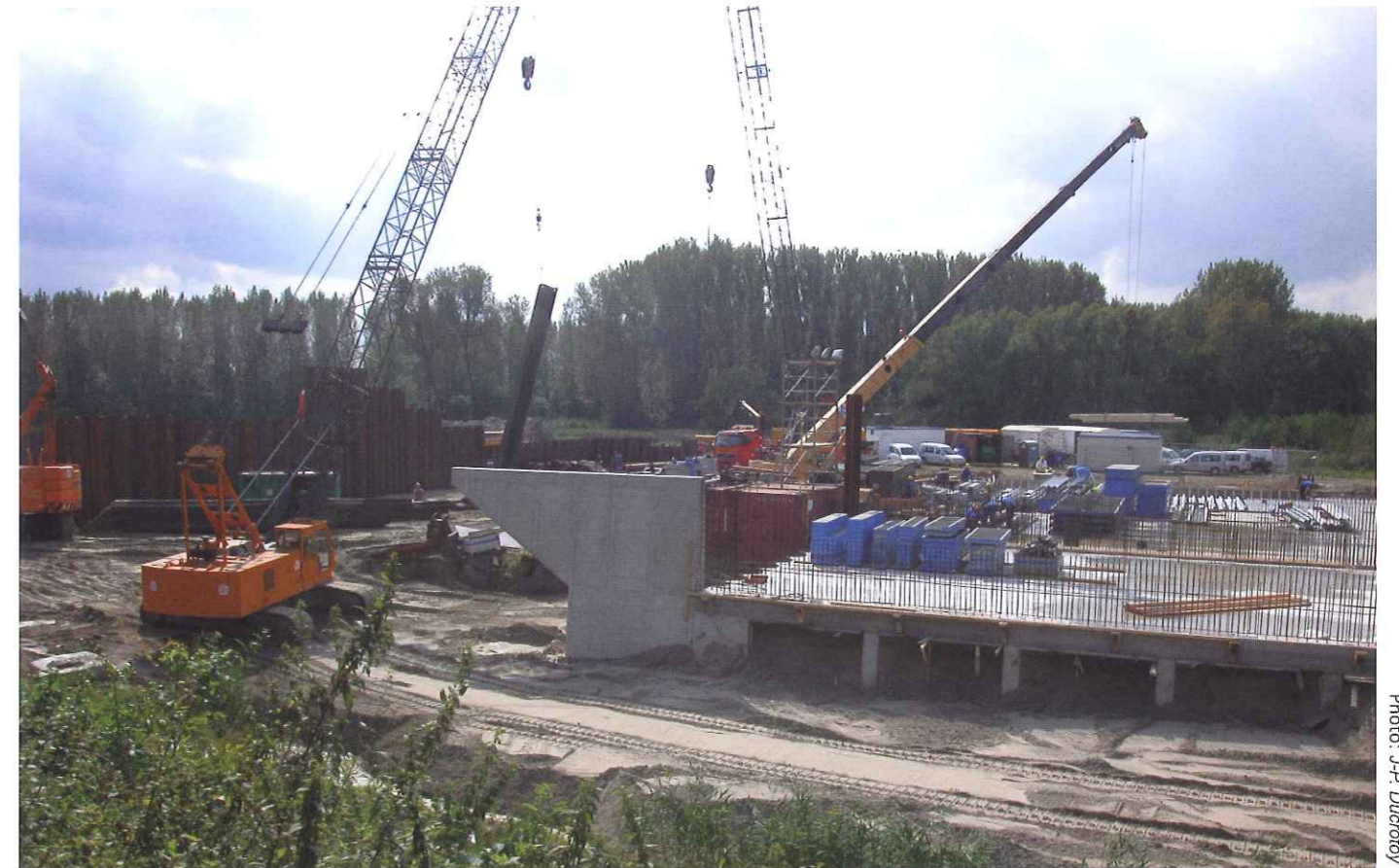
Construction of a polder under controlled reduced tide (CRT) in the Scheldt estuary, Belgium.
