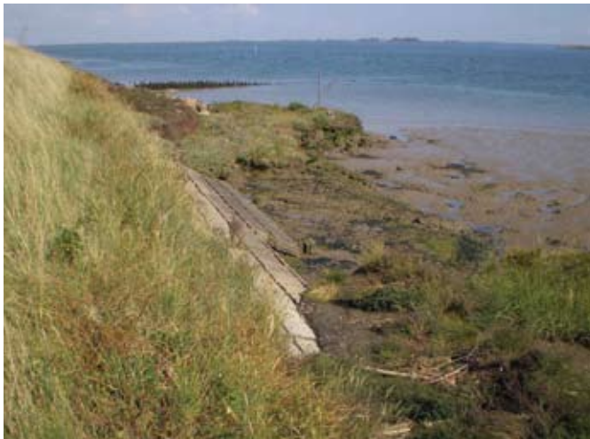
Photograph 3. Saltmarsh erosion exposing the toe of the sea wall at Wallasea Island, Crouch and Roach Estuary, Essex. This photograph shows classic coastal squeeze features: cliffed saltmarshes, lowered mudflats and undermining of sea walls.
